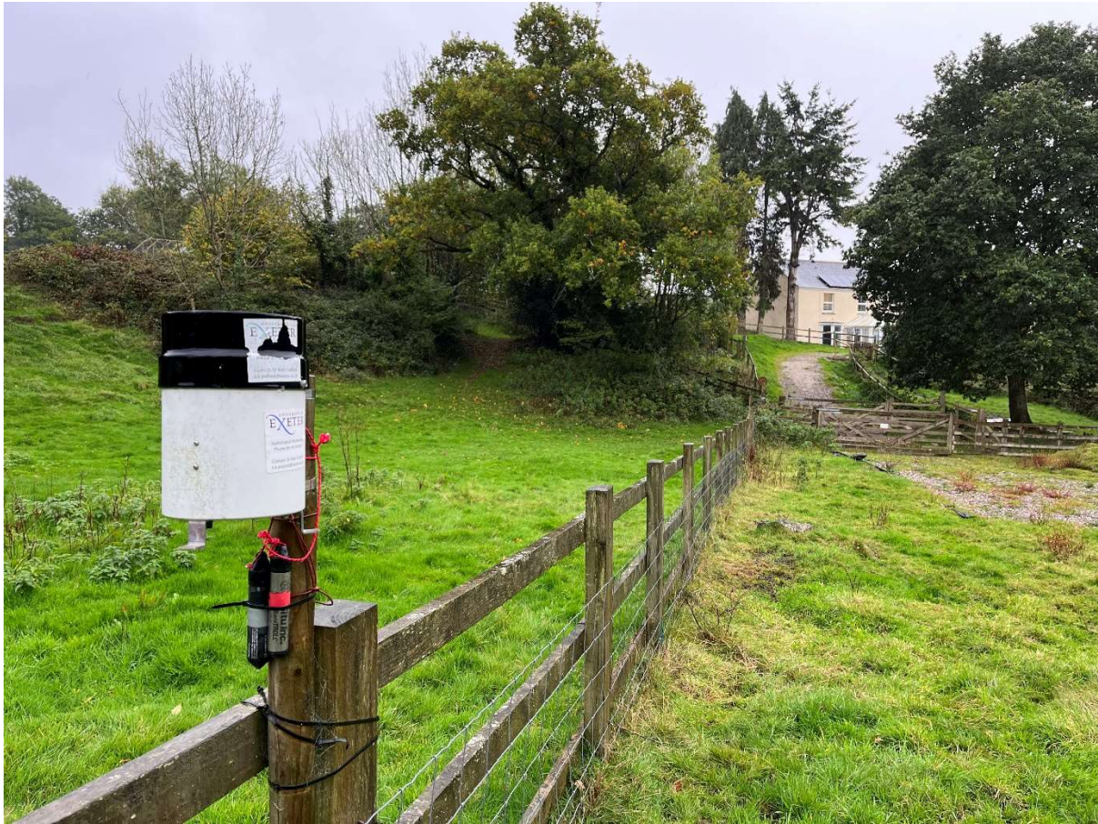
Figure 16. Rain gauge and barometric sensors installed at Poole Farm.
