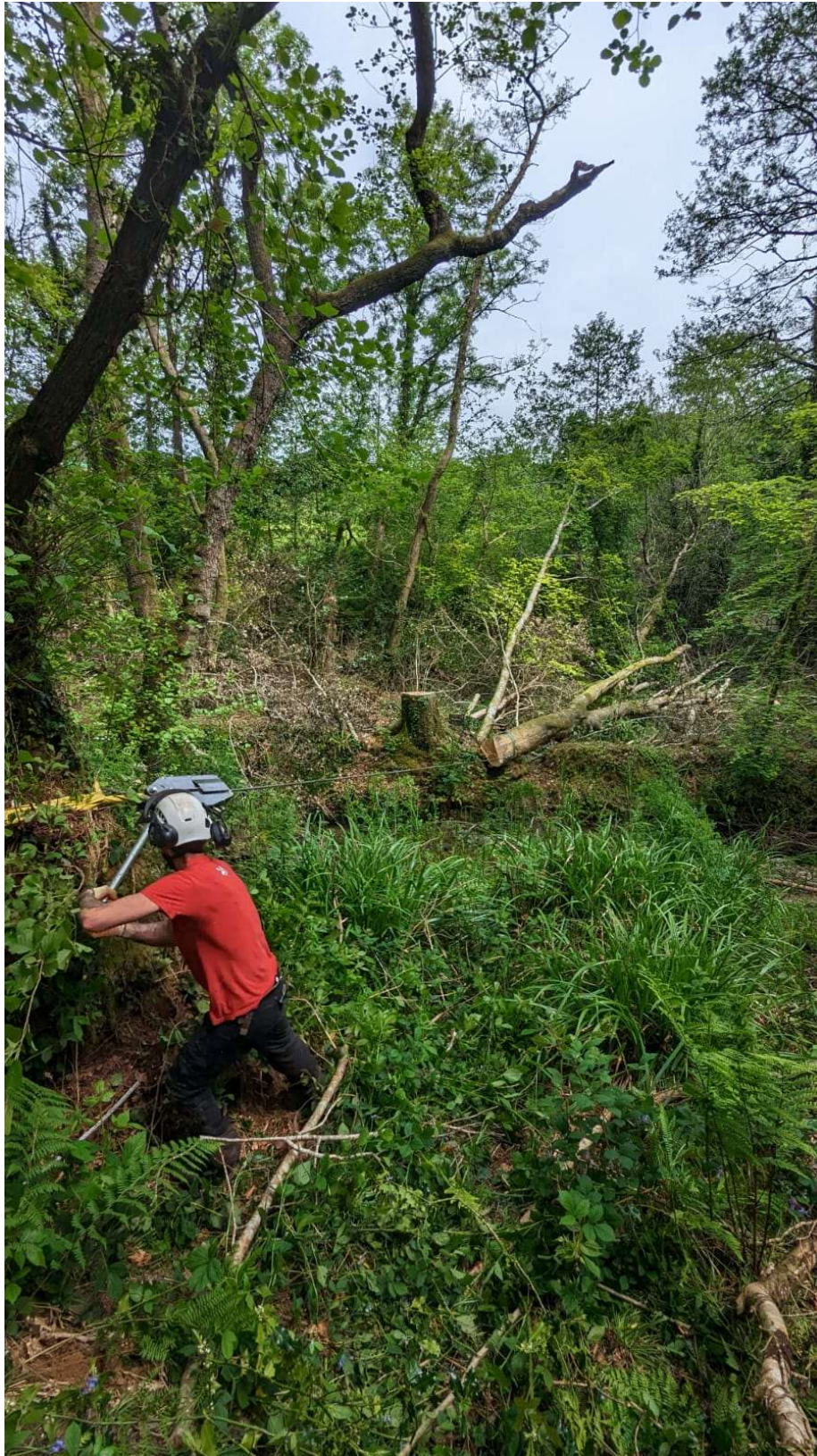
Figure 6. Work underway at the site to install NFM features. © Plymouth Natural Grid.
